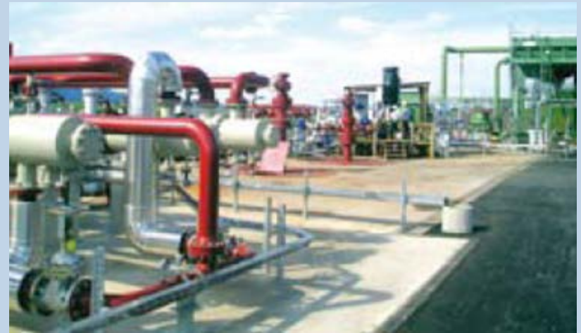
1.5 MW binary EGS power plant (Saultz-sous-Forêts, France)
