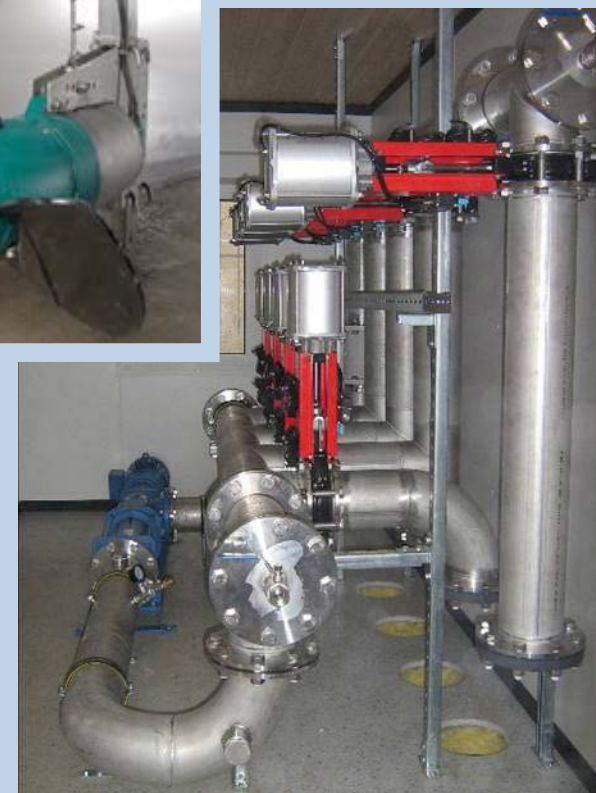
Screw pump with stainless steel piping
