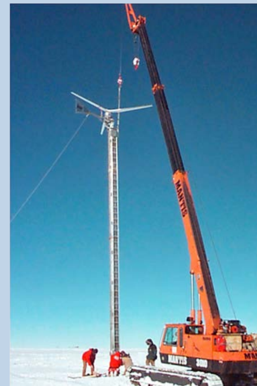
16 m tubular tower
