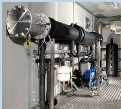
Biogas drying unit
