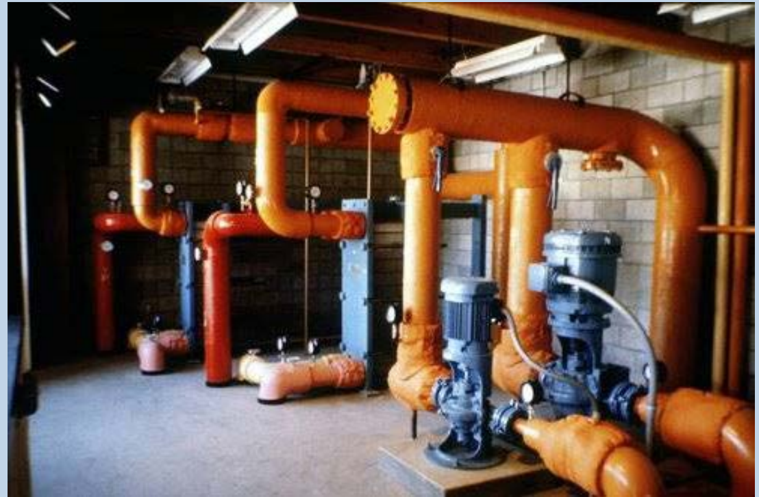
Heating exchangers and circulation pumps in a geothermal district heating system (Klamath Falls, USA)
