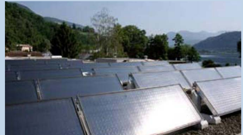
Solar panels with cushion absorbers
